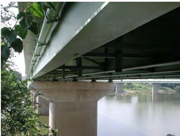
View of the underside of the eastbound U. S. 40/ National Road bridge. Source: Storrow Kinsella Associates Inc
