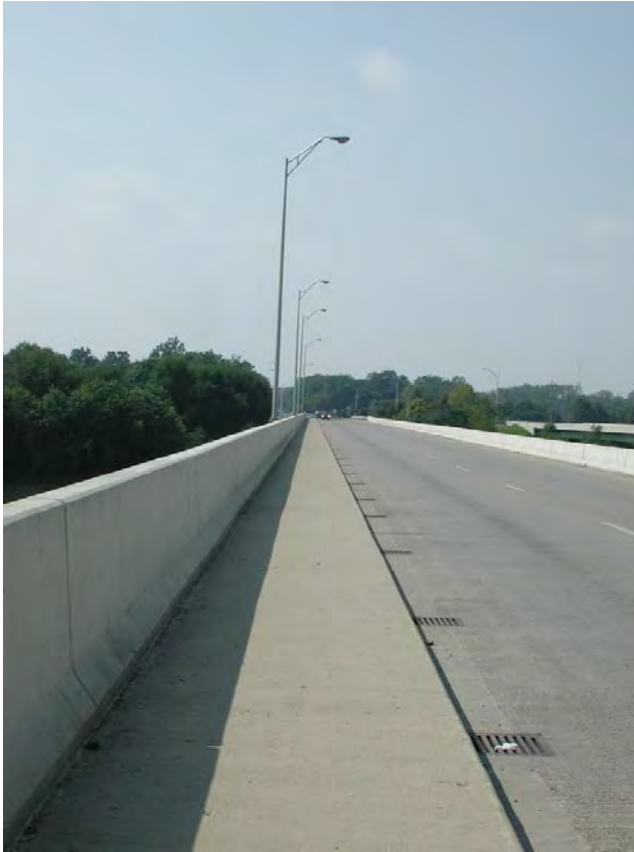
Existing pedestrian walk along south side of US 40 eastbound bridge over Wabash River. Source: Storrow Kinsella Associates Inc
